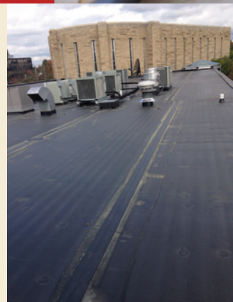
The roof over the Koegel Spiritual Center no longer leaks, thanks to repairs funded by a Foundation grant of nearly $98,000.
